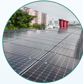
High Efficiency Solar PV System
